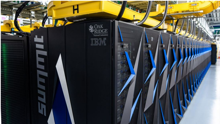
The Summit supercomputer at Oak Ridge National Laboratory, Tennessee, 2018. Photo: Oak Ridge National Laboratory. CC BY 2.0.
